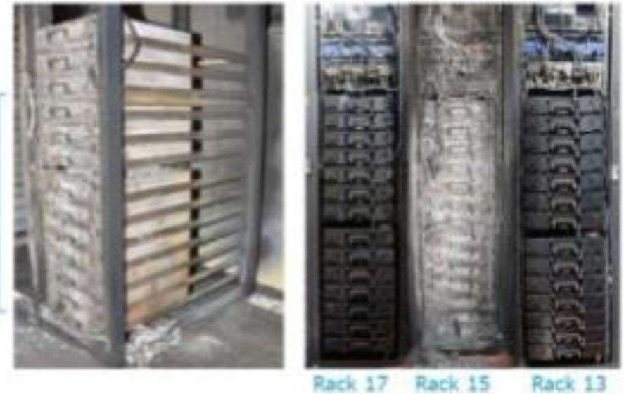
Figure 4: All modules in Rack 15 were severely damaged by thermal runaway while leaving nearby racks mostly intact (Image credit: APS) [1]
