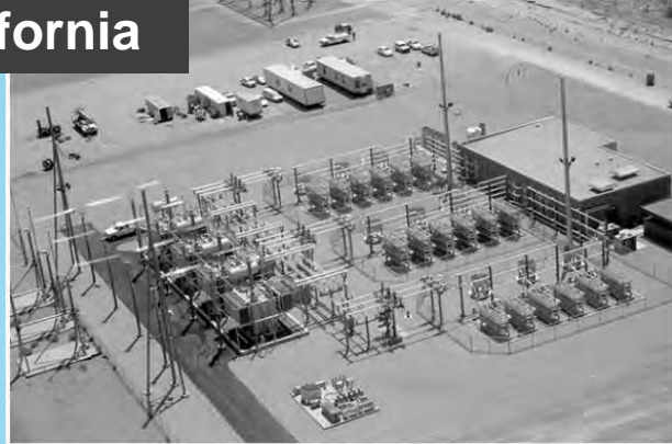
Figure 5 – 500 kV, 400 MVar SVC at Adelanto, California (by SIEMENS)
