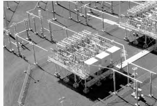
Figure 7 - Aerial view of BFA's Slatt, Oregon, 500kV TCSC (by GE)
